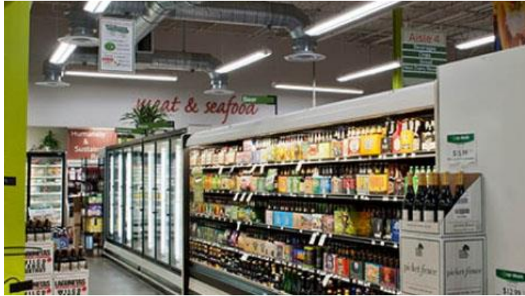
Figure 4: LED Retrofit Lighting Fixtures
