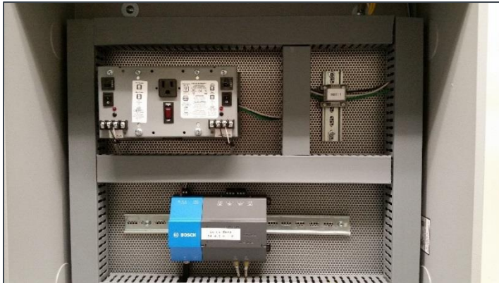
Figure 4: Tridium Building Automation System JACE
