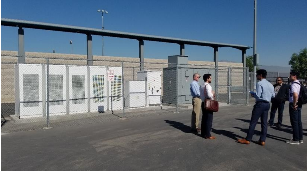
Members of the project team meet with Chino Hills Unified School District staff in front of a bank of Tesla commercial battery units at Chino Hills High School
