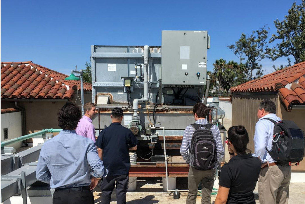
Members of the project team meet with the facilities engineer to scope the rooftop chiller at the Hilton Garden Inn Old Town San Diego
